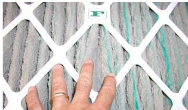
Filter Test: The 30/30 after only four months of operation.
